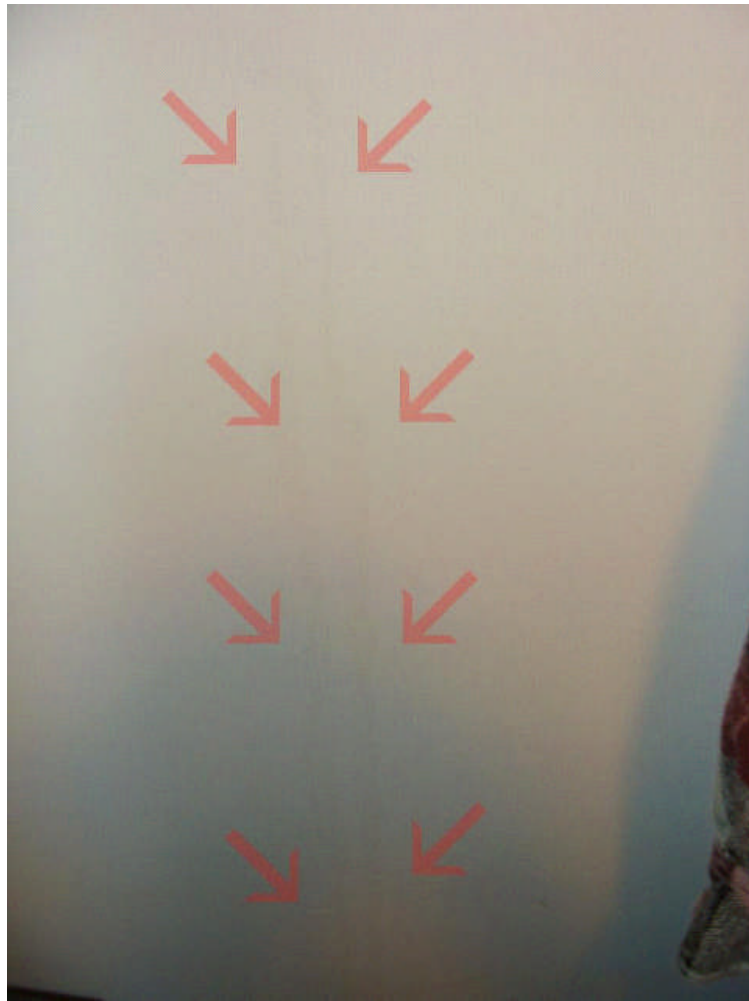
The above is a photo of stains on the closet wall.
