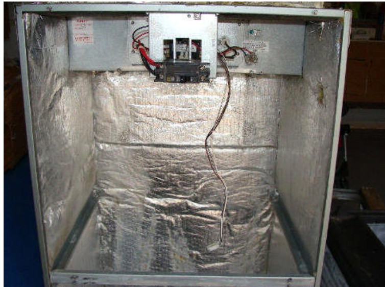
The above is a photo of the AC unit enclosure that was removed and cleaned.
