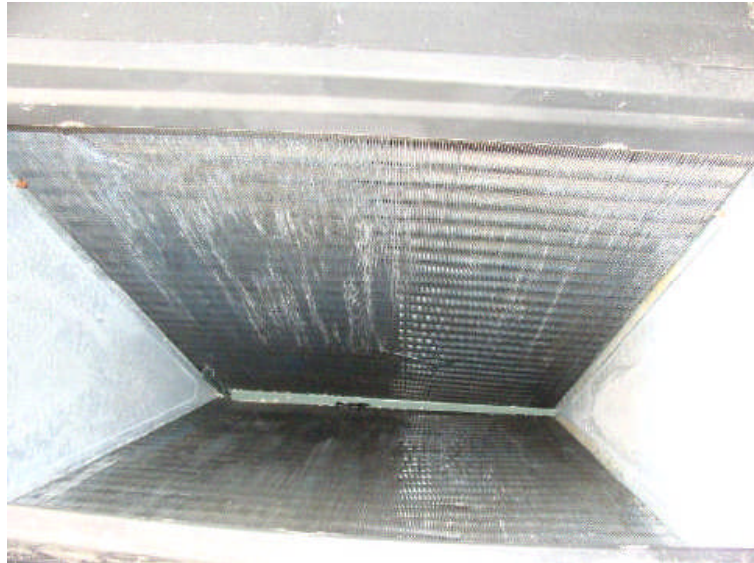
The above is a photo of the AC coils that were removed and cleaned.
