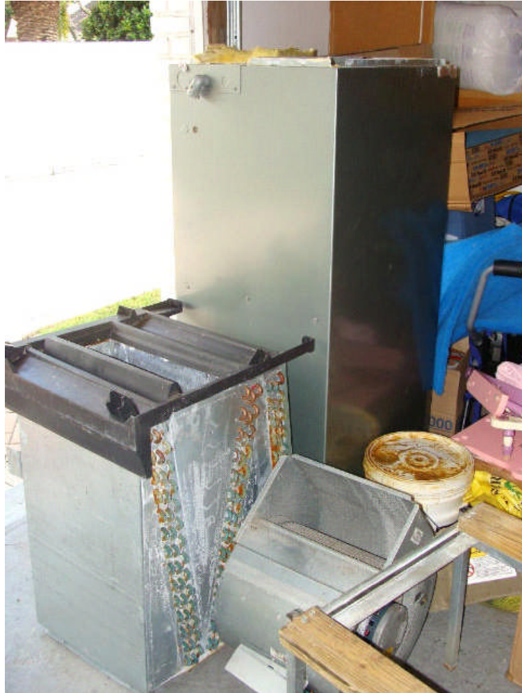
The above is a photo of the various AC components that were removed and cleaned.
